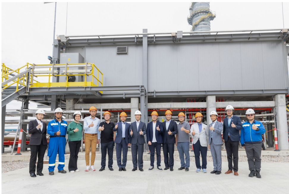
Legislators visit the new gas-fired generation unit D2 switch room, which features a raised-floor design as an example of measures taken to combat extreme weather.
