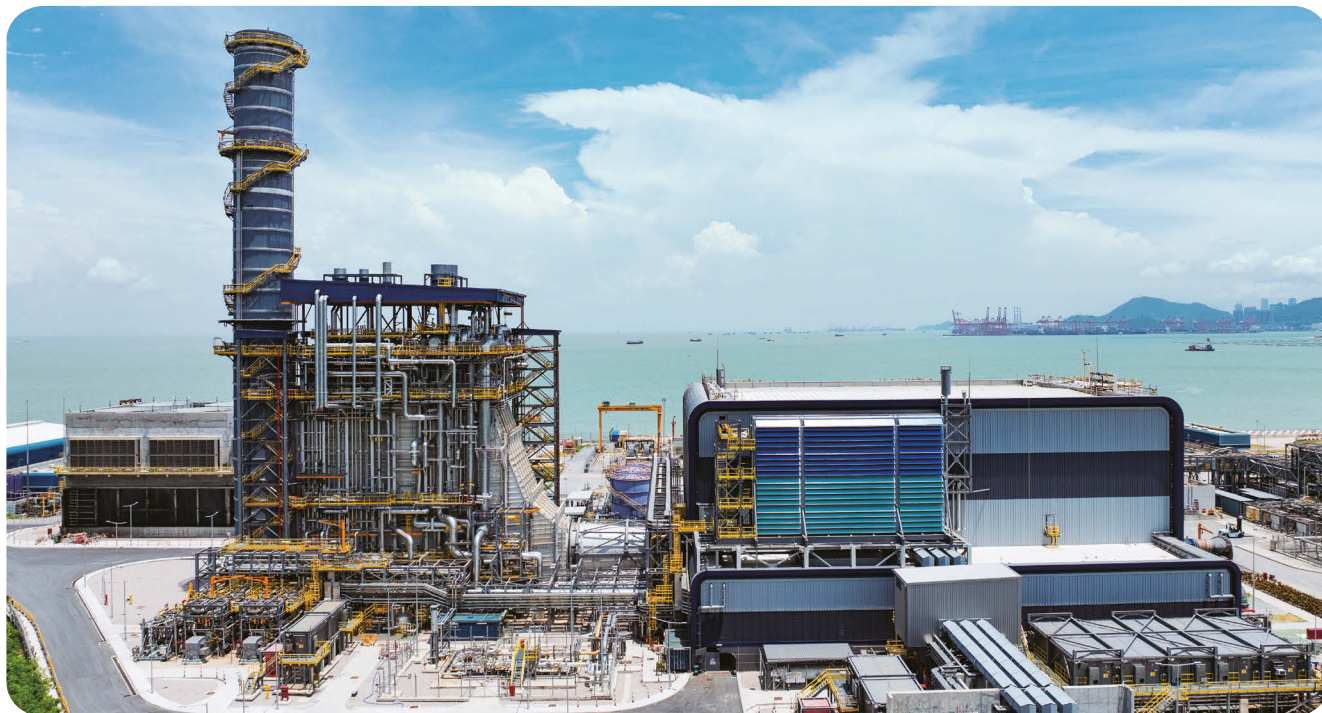
■ The new 600MW gas-fired generation unit at Black Point Power Station helps reduce the carbon intensity of electricity generation in Hong Kong, representing a major step forward for the city's energy transition.
