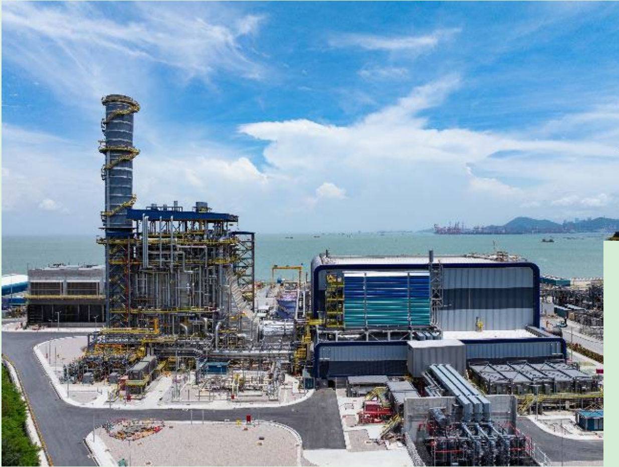
CCGT D2 gas-fired generation unit at Black Point Power Station, Hong Kong.
